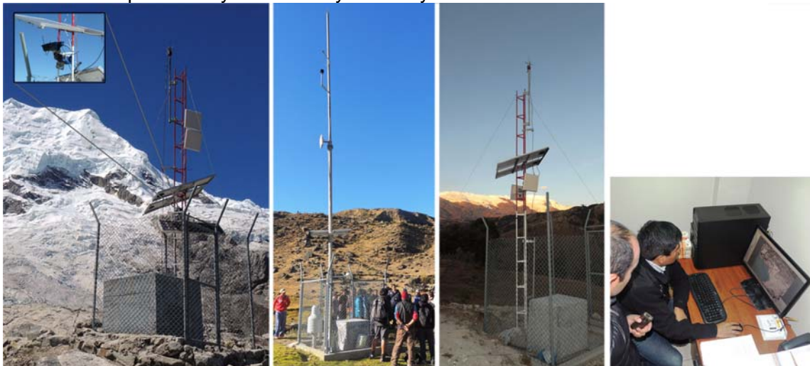
Figure 6: From left to right: Station Laguna 513 (inset showing the two cameras), Station Pampa Shonquil, Repeater Station, and main screen in the data center at the municipality of Carhuaz. Photos by CARE Peru.
